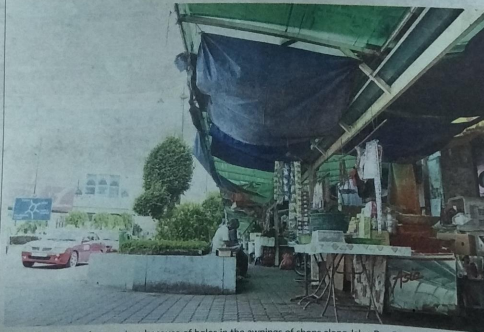
Plastic sheets have been put up because of holes in the awnings of shops along Jalan Pos Baharu that are in dire disrepair.
