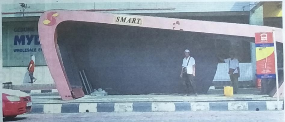
Work on the Smart Selangor bus stop in Jalan Pos Baharu stopped halfway and the shelter already looks dilapidated.
